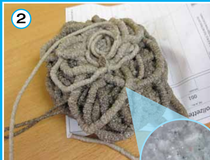
BBU purging clearly shows carbon evident in purge
